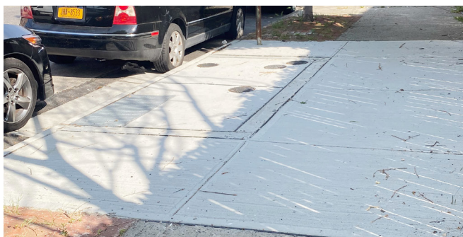
Infiltration Basin with Concrete Top
