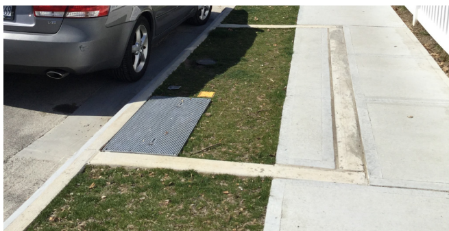
Infiltration Basin with Grass Top
